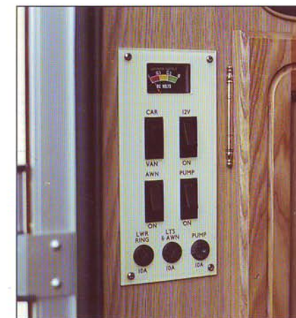
The Control Panel is conveniently located by the door
